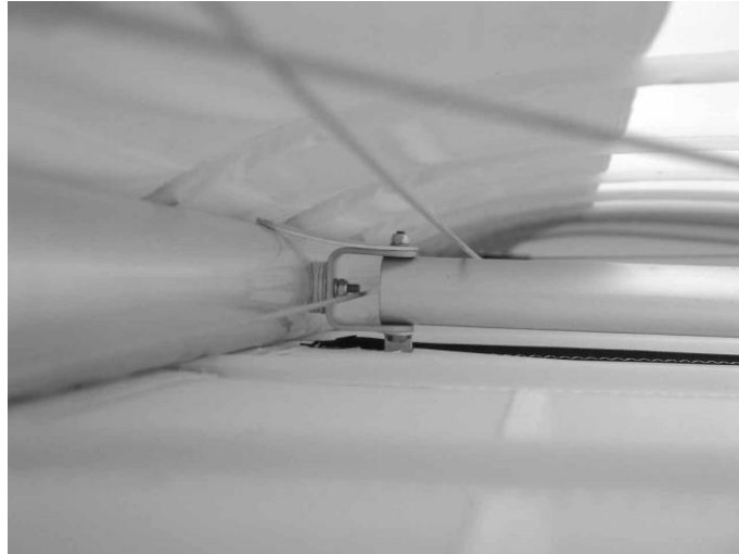
Figure 148 cable routed through U-bracket.
