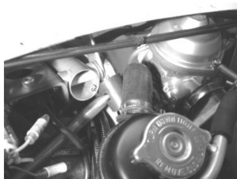
Figure 212 expansion tank and rubber elbow.
